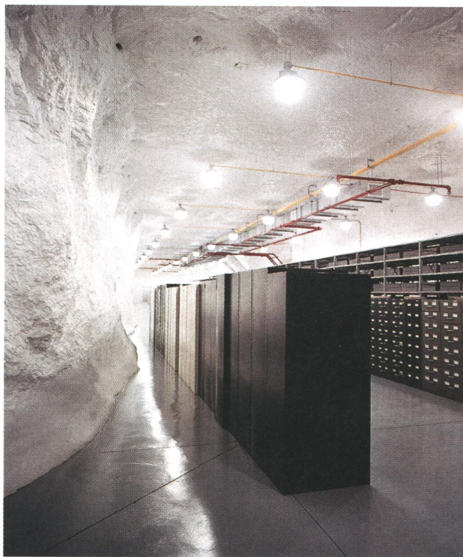
A section of newly installed file cabinets for the Corbis collection, part of its cache of 11 million images.
