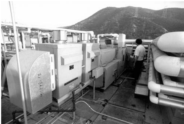
Cargocaire continuous desiccant dehumidifiers and other air-handling equipment for one of the film storage vaults.
