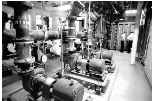
The refrigeration machinery room. To avoid cooling and dehumidification failures, all systems are fully redundant.
