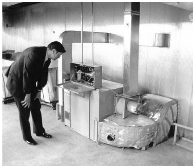
A Cargocaire dry desiccant dehumidifier attached to a color motion picture film storage vault (maintained at 25% RH and 37°F [2.8°C]) at the Library of Congress facility in Landover, Maryland, near Washington, D.C.
