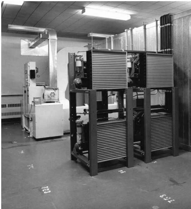
Four refrigeration compressors operating in a redundant mode cool the vault at the National Archives of Canada. Behind the compressors is a Cargocaire dry-desiccant dehumidifier that maintains 28% RH in the vault.
