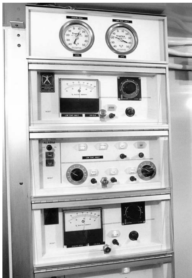
Linked to temperature and relative humidity controls, an automatic alarm system alerts security personnel if conditions inside the vault exceed preset limits.
