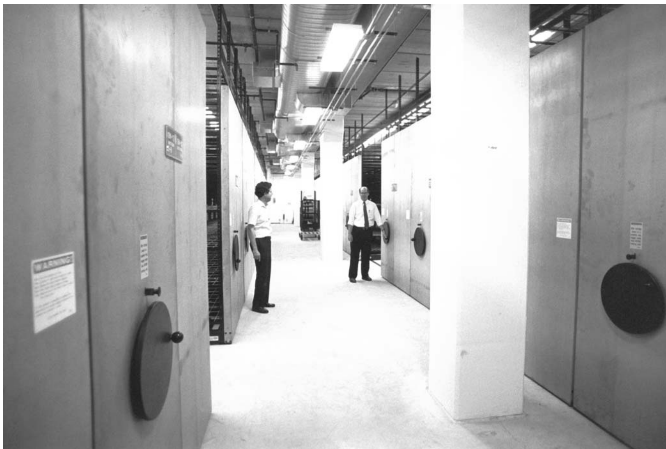
One of the three film storage vaults in the new Warner Bros. high-security motion picture cold storage building on the Warner Bros. studio lot in Burbank, California. The color film vault, which is maintained at 35°F (1.7°C) and 25% RH, and the other vaults were operating and in the final phase of testing when this photograph was taken on October 8, 1992. Warner Bros. began moving its film collection into the vaults a few weeks later. Shown here in the larger black-and-white film vault, which, like the two other vaults in the building, is equipped with movable shelving that permits high-density film loading, are John Belknap, manager of Film Vaults/Assets, and Bill Hartman, manager of Asset Inventory Management and Research in Corporate Film Video Services at Warner Bros. The $9-million cold storage facility was designed under the direction of Peter R. Gardiner, vice president of Operations in Corporate Film Video Services at Warner Bros. (a division of Time Warner Inc.). See Chapter 9 for additional discussion of the film preservation program at Warner Bros.
