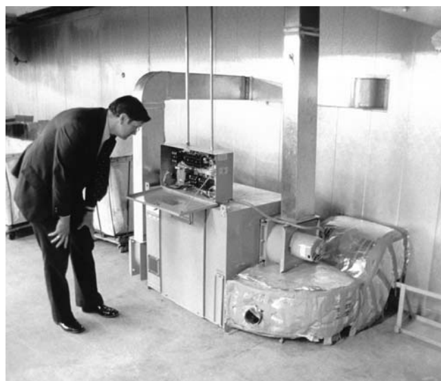
A Cargocaire dry desiccant dehumidifier attached to a color motion picture film storage vault (maintained at 25% RH and 37°F [2.8°C]) at the Library of Congress facility in Landover, Maryland, near Washington, D.C.
