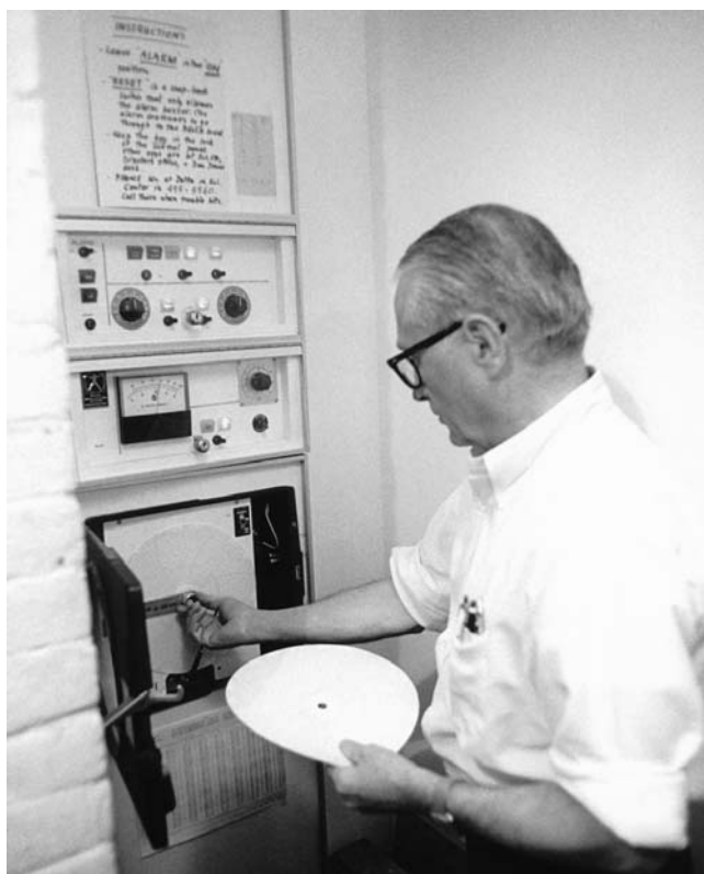
Jones changes the charts in the recorder for temperature and humidity in the control panel outside the vault door.
