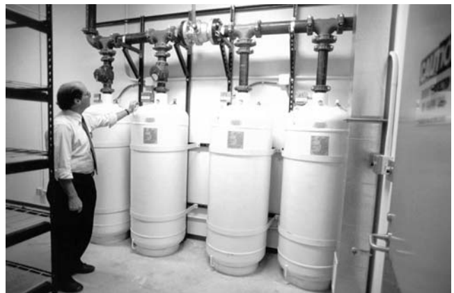
Haylon gas fire-suppression systems are provided for each of the film vaults in the fire- and earthquake-resistant building. Security systems are monitored 24 hours a day.
