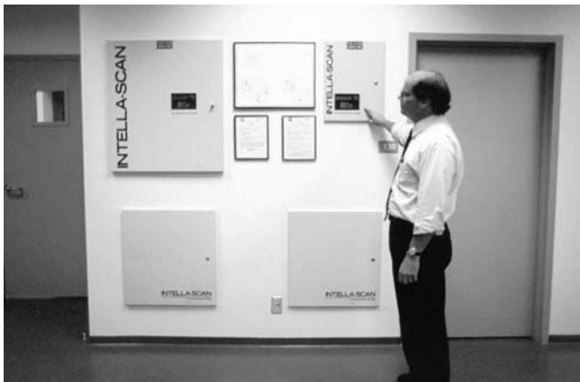
The building is equipped with an advanced fire-detection and intrusion alarm system. Access to film vault areas is electronically restricted to certain key personnel.
