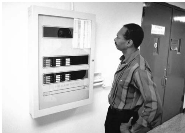
Film vault manager Sam Tyler regularly checks the fire alarm control panel. Sensors in each of the 96 vaults will trigger an alarm if there is a mechanical failure in the cooling equipment or if smoke or fire is detected. Smoking is absolutely forbidden in the vault area.
